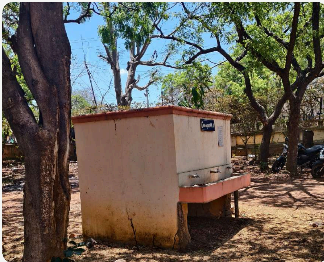
Image 12: Handwash Facility, Koppanappatty PHC, Pudukottai
