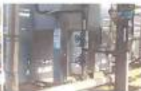
Anion Rinse Water Pumping Pit
